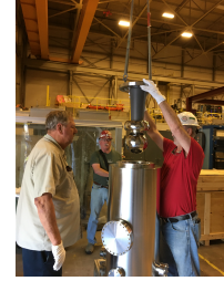
Due to its share weight (~60 lbs), the insulator-electrode assembly was installed into the test chamber using a crane. The electrodes were mechanically polished to mirror finishing in a tumbler barrel polisher 5 .
