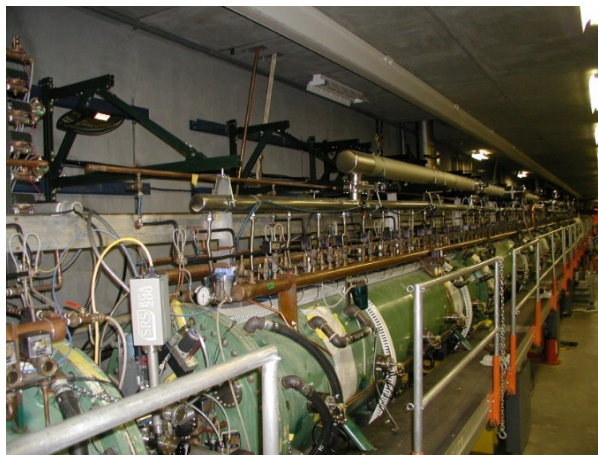
Figure 1: LANSCE DTL modules.
