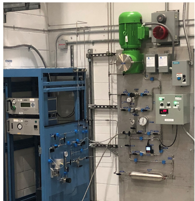
Figure 3: Installed helium gas analysis recovery system.
